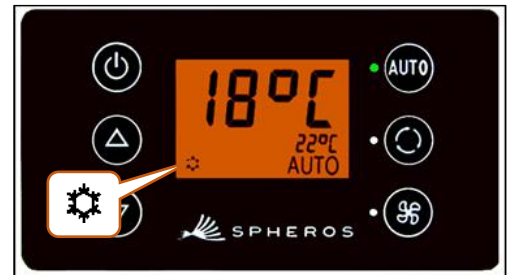
Figure 6 - SC600 Auto mode activated, Cooling mode
