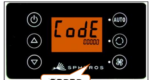
Figure 12 - 00000 access code entry
